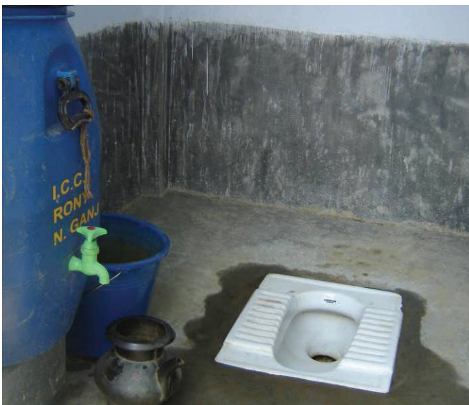
A hygienic latrine with hand-washing facilities.
